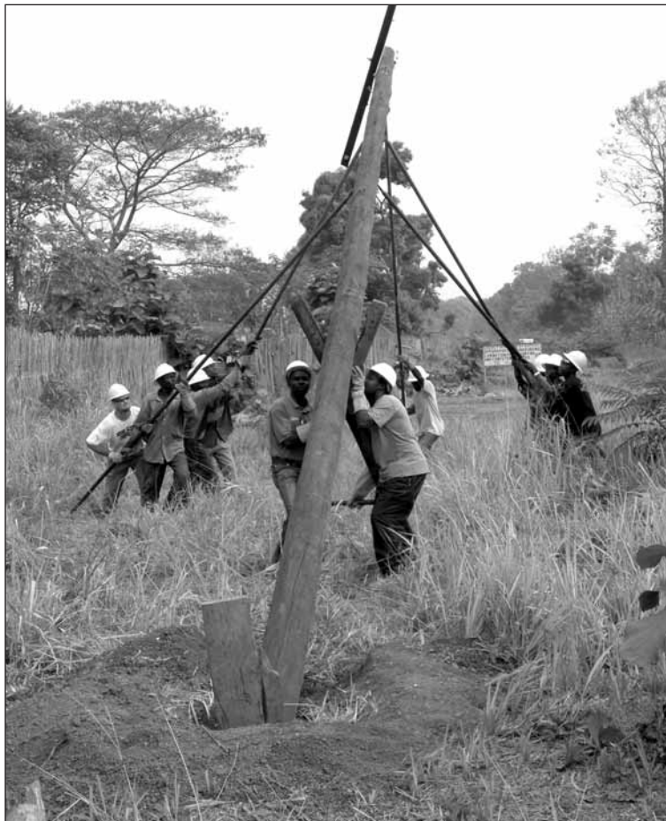
BEC Lineman Steve Baumgartner, on the far left, helps Yei utility workers raise a power pole. The line construction is completely manual since the local cooperative has no access to bucket trucks or digger derrick trucks. The men are using pointed pike poles to help push up and steady this 45-foot power pole to help carry a three-phase electrical line.
