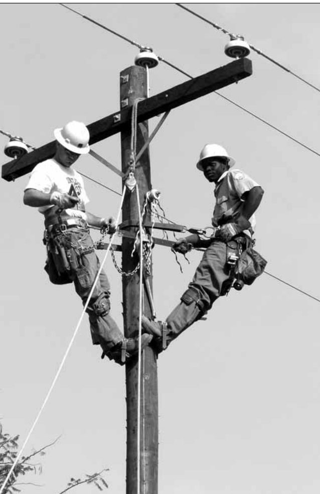
Lineman Jamie Conrow works atop a power pole in Yei, Sudan, with local cooperative lineman Hakim James. Six American linemen and local linemen power streetlights and build a three-phase line to power a school, medical center and church.
