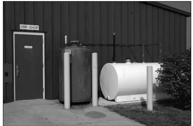
Used oil from Boone Electric's vehicle fleet pumps directly to these storage tanks. It will be used in an oil-burning furnace to heat the Vehicle Maintenance Facility each winter.
