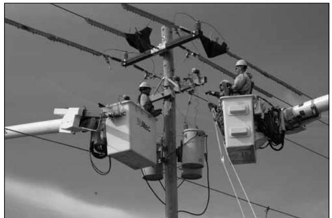
Linemen work each day with a dangerous product. These linemen have used every precaution, including wearing insulated sleeves and gloves, as well as covering and wrapping the energized lines with insulators and rubber covers.
